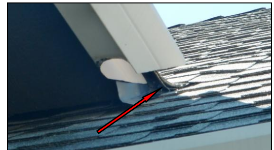
Photo 2RF: This gutter is cut to allow water to drain directly on shingles. Recommend piece of metal flashing underneath.
