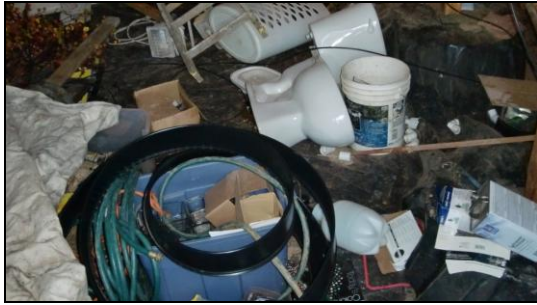
Photo 3STR: This debris in crawlspace should be removed.
