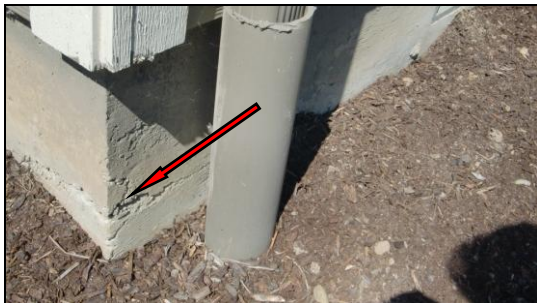
Photo 1STR: Minor spalling of this corner of home. Recommend parge/seal with concrete mixture to mitigate moisture penetration.
