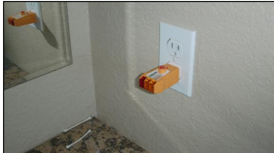
Photo 2ELE: This master bathroom outlet did not function when tested.
