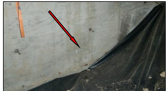
Photo 2STR: Settlement seams developed in the foundation wall in the crawlspace. This is typical and appears to have no structural significance.
