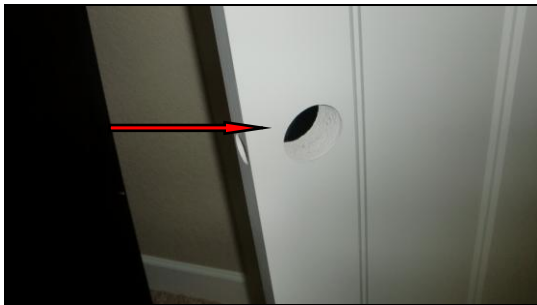
Photo 3INT: Guest bedroom closet door is missing a handle. Easy fix.
