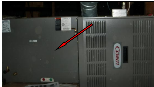
Photo 1AC: This unit is a supplemental heat pump/air handler system designed to reduce energy costs for cooling and heating. The primary system is gas furnace. The system will need an outside condenser unit and lines connecting it for operation. This is discretionary. Good system to have.
