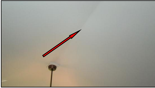
Photo 1INT: There are hairline cracks in apex of vaulted ceiling in living room. This is a typical issue with drywall and is not a major concern.
