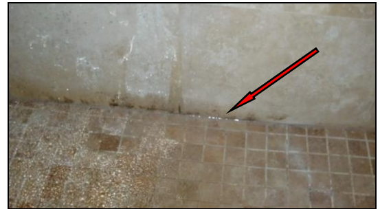
Photo 2INT: Mildew is accumulating at the base of this shower in master bathroom. Recommend clean this.
