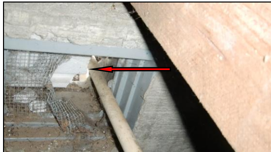
Photo 1INS: This vent screen is torn away to allow TPR piping to exterior. This hole should be covered to prevent vermin entry.
