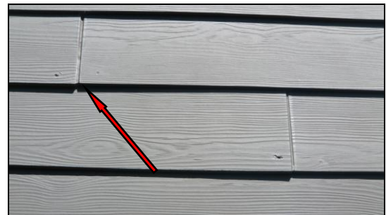
Photo 2EXT: These panels should be better secured to house sheathing.
