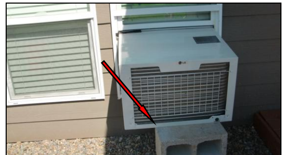
Photo 2AC: This mount is not recommended. The unit should be sitting on more of the concrete block.
