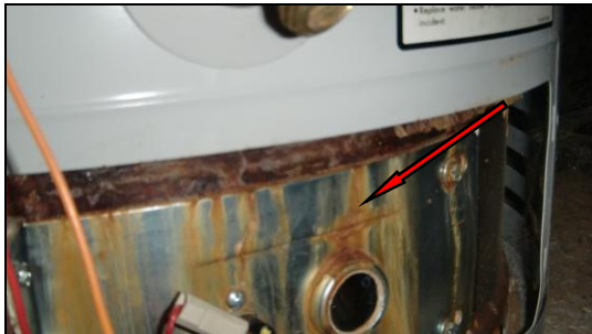
Photo 1PLU: Unusual rusting is taking place around the water heater burner unit. Recommend service to determine problem.
