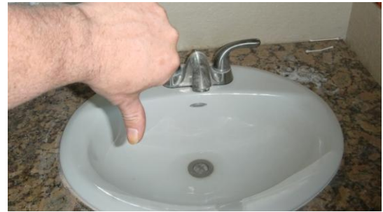
Photo 2PLU: Both sink stoppers are inop. Right side sink will not drain water.
