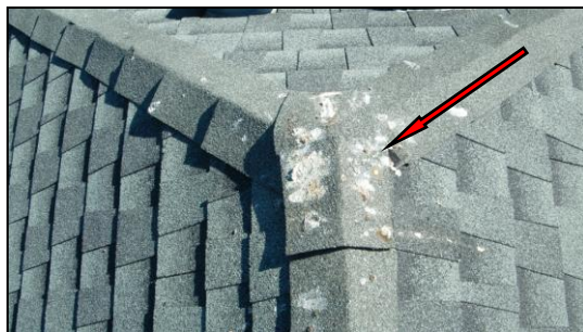
Photo 1RF: This problem may have been at installation with roofers providing extra nails to secure shingle. This is topmost ridge cap.
