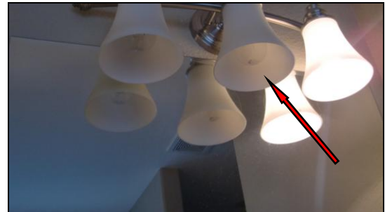
Photo 1ELE: Lights did not operate.
