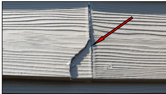
Photo 1EXT: Several panels are cracked in this way. Repair is discretionary. Recommend caulk and monitor.
