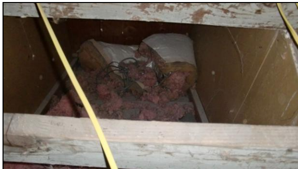
Photo Attic: This enclosed stairwell to the attic (near laundry room) may be a cold spot.
