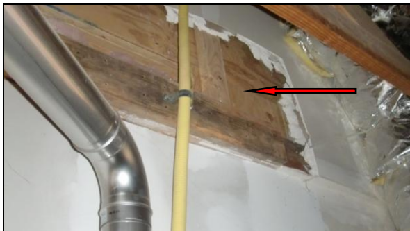
Photo 1EXT: The installation of drywall over wood framing connected to the home should be completed in the garage.
