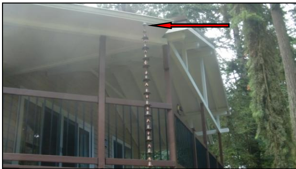
Photo 1RF: This drip spout should be replaced with a conventional downspout to keep water away from the home.
