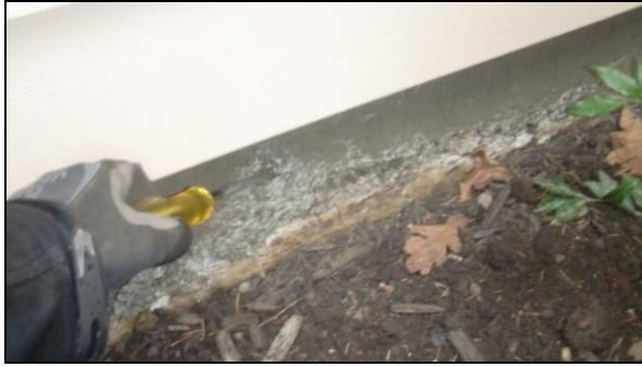
Photo 3STR: Slight, localized deterioration of the base of this foundation should be repaired with a concrete parge to keep water out.
