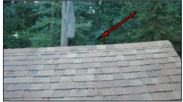
Photo 4STR: There is slight sag at the ridgeline. This is common for rafters but should be monitored.
