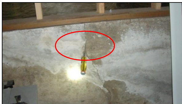
Photo 1STR: This settlement crack runs diagonally and is larger than typical. This crack should be sealed on the exterior and monitored for any potential widening.
