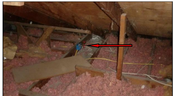
Photo 2ELE: These exposed wires should be properly terminated in the junction box. In Attic above the living room.
