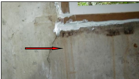
Photo 1INT: Evidence of moisture penetration was observed beneath a rear basement window.
