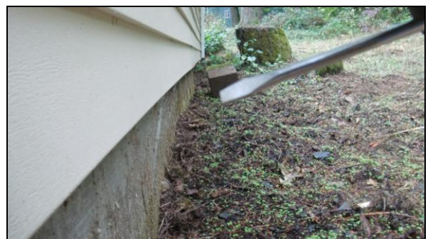
Photo 2STR: Outside view of this wall shows signs of bowing inward and outward. This may be an original flaw in setting the concrete. Recommend water be properly drained away.
